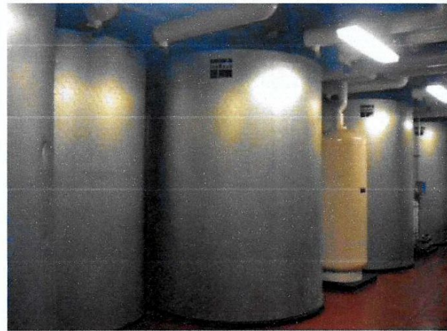
CALMAC IceBank energy-storage tanks installed at Rockefeller Center.
